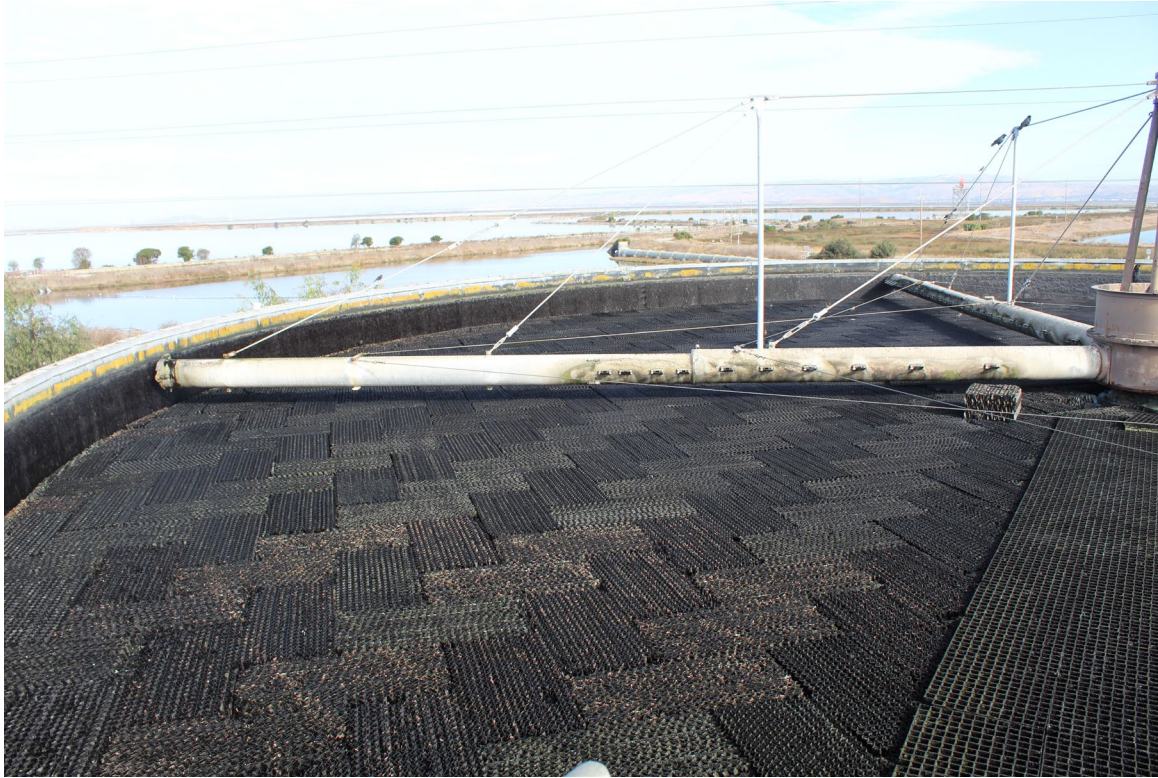
Replaced Media in Fixed Growth Reactors
