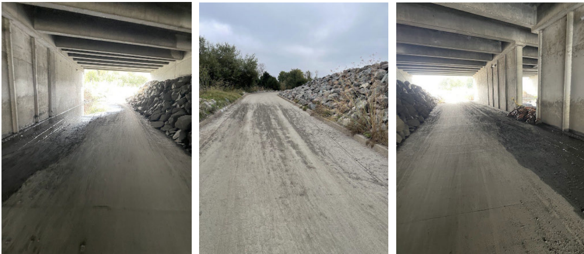
Figs. 1-3: Photos of the Trimble Road underpass, taken around 10/24/2025, roughly two weeks after the underpass initially flooded. The trail is partially dry and could be partially cleaned, but no cleaning occurs until all water has evaporated and mud has fully caked. Tracked-out mud is a fall hazard in dry conditions and becomes more dangerous with any precipitation.
