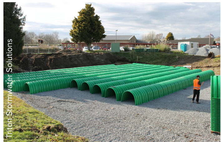
Subsurface Infiltration Gallery
