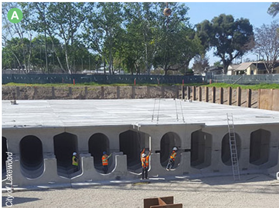
City of Lakewood Example of Subsurface Infiltration Chamber under Large Green Space at Bolivar Park in Lakewood, California
