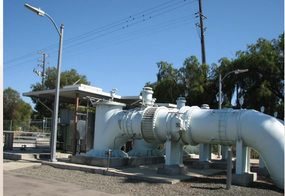
Rincon I Storm Pump Station
